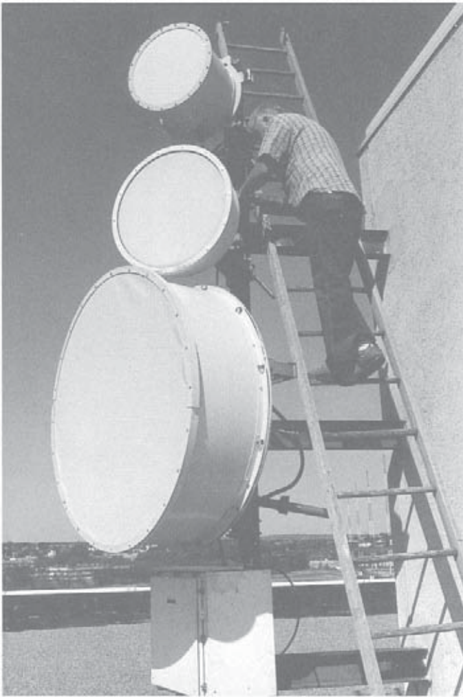
Fig. 7. Roof-mounted microwave antennas provide point-to-point broadband communications in an office park.
